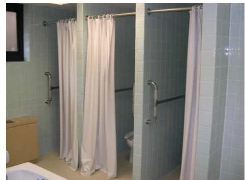
TYPICAL GANG TOILETS (NOTE: NON COMPLIANT ACCESSIBILITY MEASURES)
