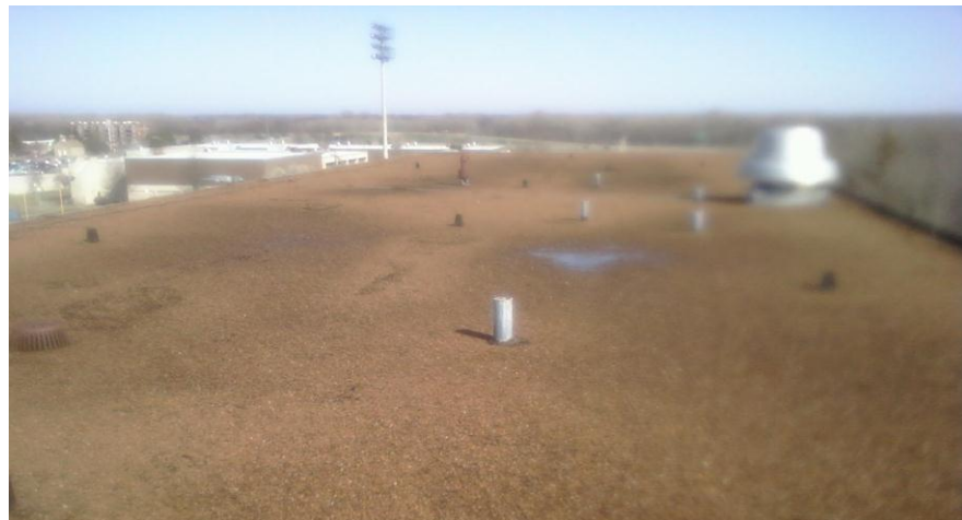
EXISTING BUILT UP BALLASTED ROOFING SYSTEM NOTE THE PONDING
