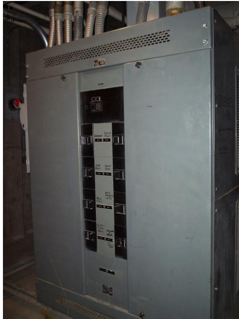
EXISTING FEDERAL PACIFIC MAIN DISTRIBUTION CENTER (NOTE: REPLACEMENT PARTS ARE NO LONGER MANUFACTURED)
